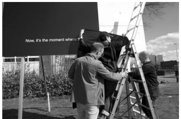
INSTALLATION DE ALL OF THEM HAVE A PROMISE , EXPOSITION COLLECTIVE D'AFFICHES DANS HEERLEN, 2021 © GREYLIGHT PROJECTS
